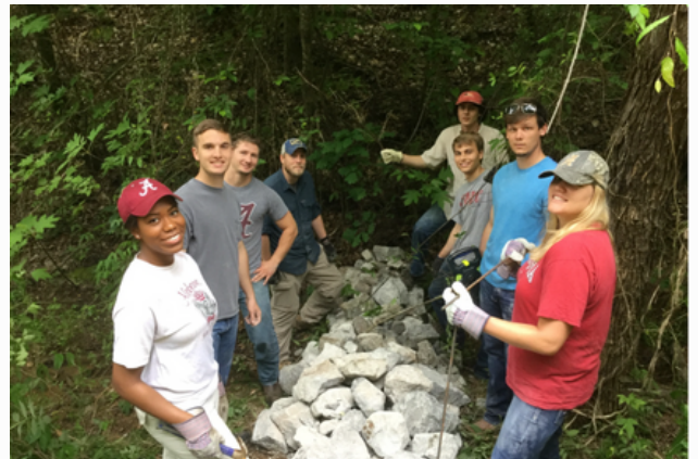
Students build a dirt-road sediment detention pit bmp for sediment control in Fayette County
